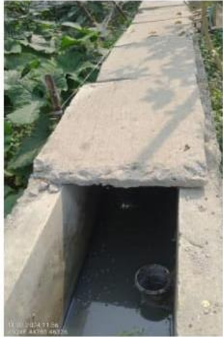
Drain carries Grey water
