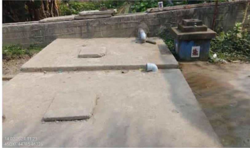
Water comes into ABR
