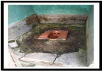
Broken floor & seat
