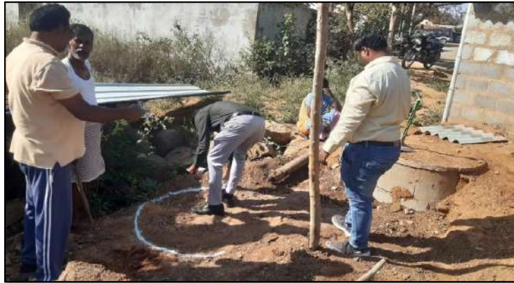
Site selection for Retrofitting of toilet single pit to twin pit in Telangana
