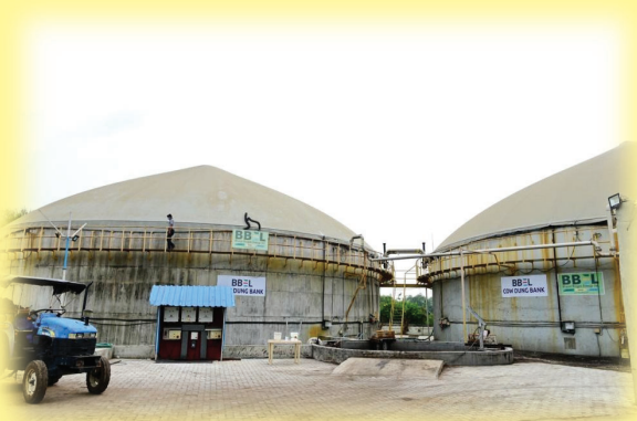
Umreth, Anand, Gujarat Entrepreneur-led central anaerobic digester model
