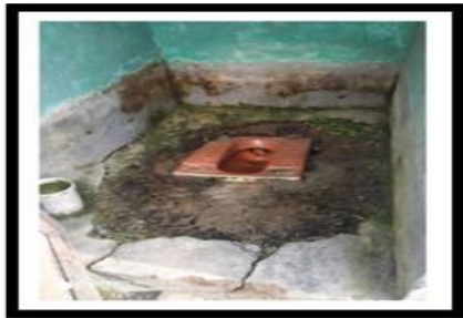
Broken floor & seat
