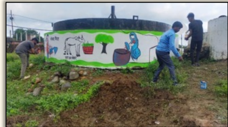
Gobar Gas Plant at GP Mendori of Phanda Block
