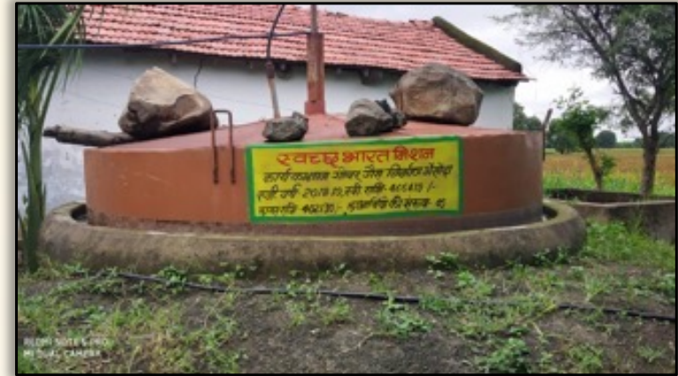
Gobar Gas Plant at GP Bhensoda of Berasia Block
