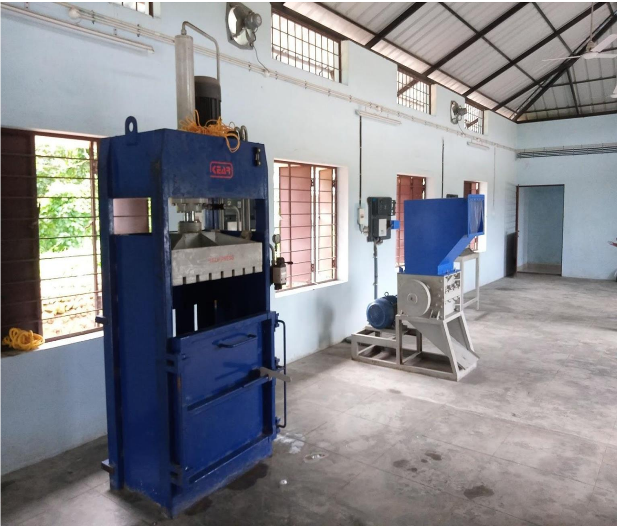
Resource Recovery Facility in Mundur BP in Palakkad
