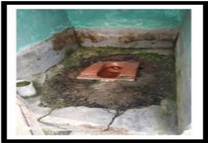
Broken floor & seat
