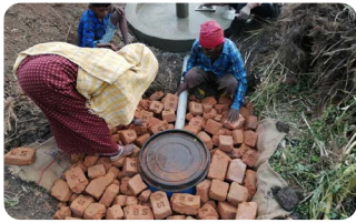
17,51,285 community soak pits
