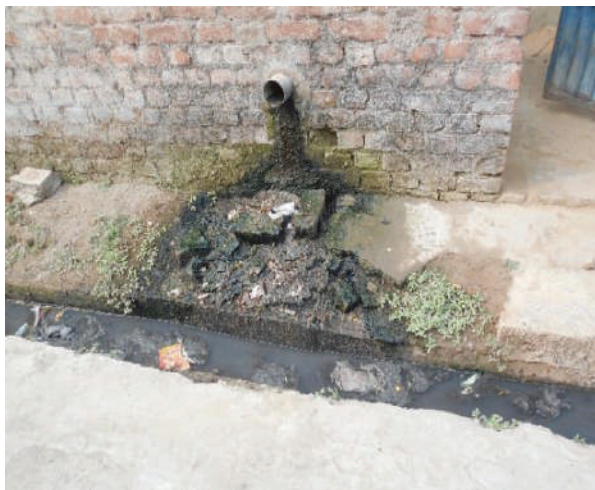
Black water from Septic tank
